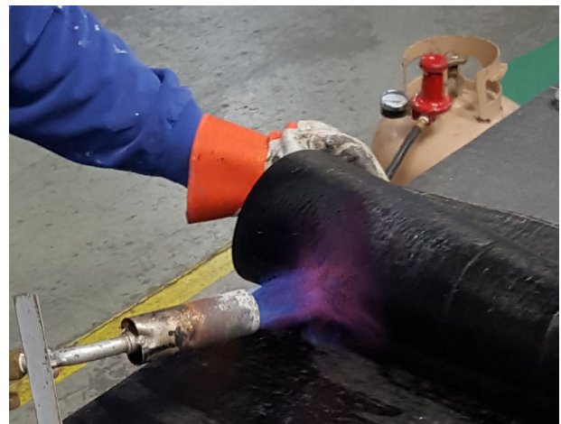
Torch applying heat to mod bit waterproofing membrane. Consult the membrane manufacturer for specific installation guidelines.
